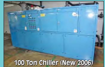
100 Ton Chiller (New 2006)
